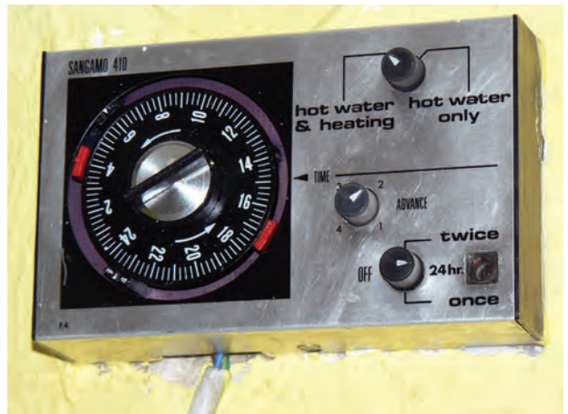
Cable sheath not taken inside metallic enclosure
