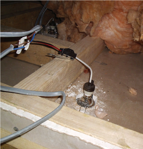
Unsatisfactory electrical connections
