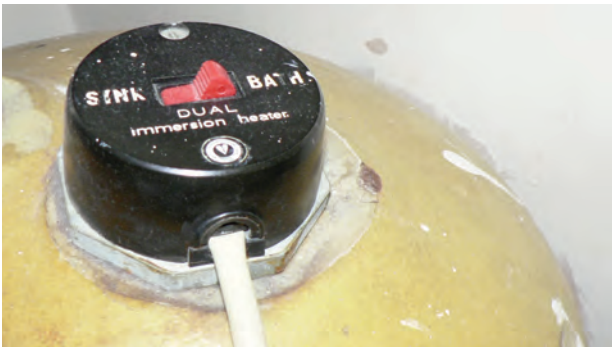
Older immersion heater without thermal cut-out
