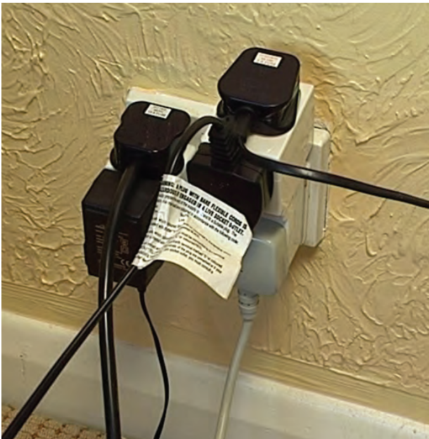
A potentially overloaded socket-outlet
