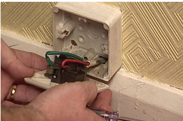
Inspecting a socket-outlet
