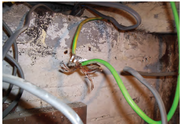
Absence of a reliable means of earthing
