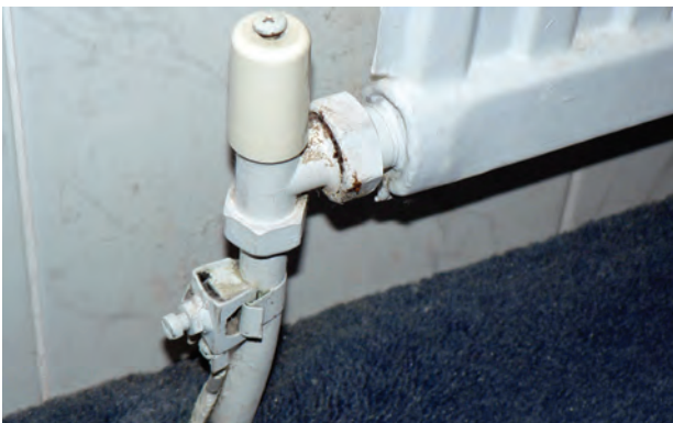
Unmarked bonding conductor
