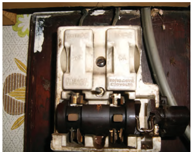
Double-pole switch with fuses in each pole
