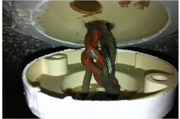
Crumbling vulcanised rubber insulation
