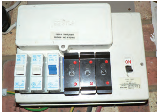
Consumer unit with circuit-breakers and fuses
