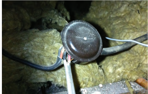
Cable sheaths not taken inside non-conducting enclosure
