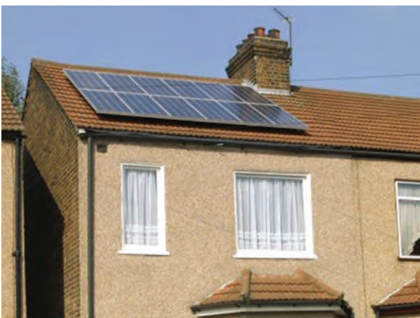
Photovoltaic installation (Photo courtesy Energy Saving Trust)
