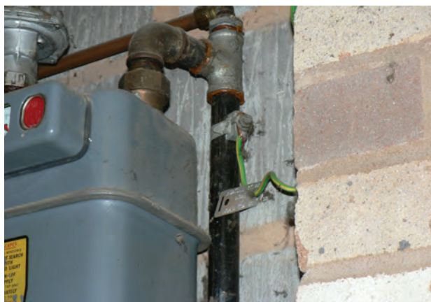
Main bonding connection not made before branch pipework
