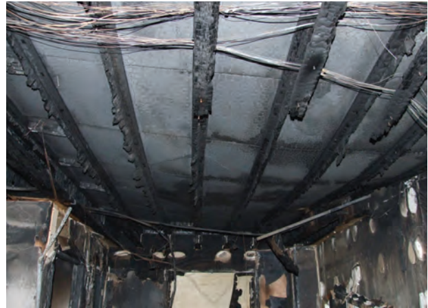
Floor above in danger of collapse (Photo courtesy of Greater Manchester Fire & Rescue Service)
