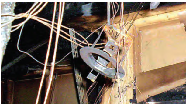
Result of a downlighter fire (Courtesy of Manchester City Council - Building Control)
